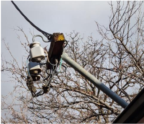
Image 1: Reported as weathered timber batten
