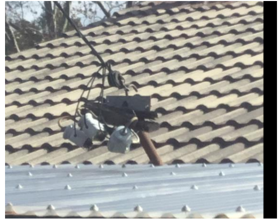
Image 4: Reported as damage timber batten
